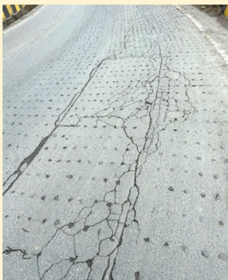
(Picture 22: Example of low temperature cracking of Mastic Asphalt in NH-110, because of snow fall during February, 2022)
