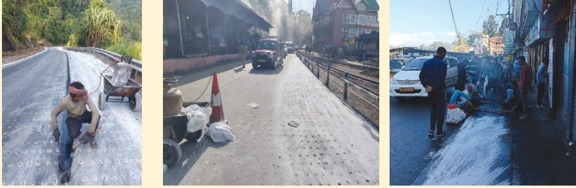
(Picture 23: Some photographs of recent execution of Mastic Asphalt in NH-110, with VG-40 as binder which performed excellently)
