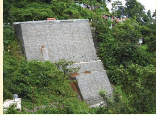
(Picture 12: After restoration, S3 spot with a height of RE structure of 38.7 Mt.)
